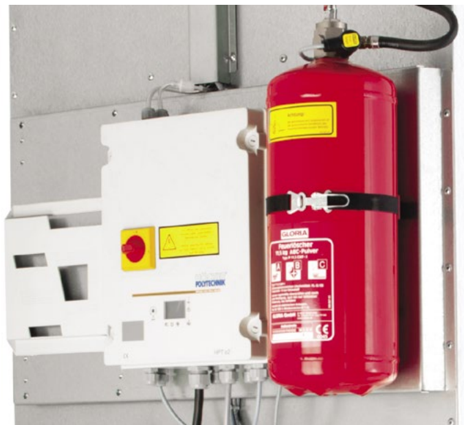
Fig. below: PLC-control, automatic fire suppression system
