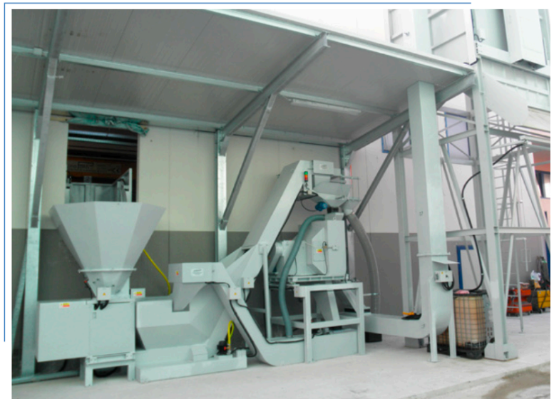
Swarf crushing and spinning plant with silos
