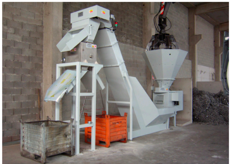
Automatic crushing system equipped with magnetic separator
